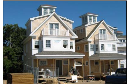
HERRING COVE VILLAGE-PROVINCETOWN PHASE I: BUILDINGS 1&2 OF 11 UNITS DESIGNED BY: MCMAHON ARCHITECTS FOREMAN: STEVE O'BRIEN
